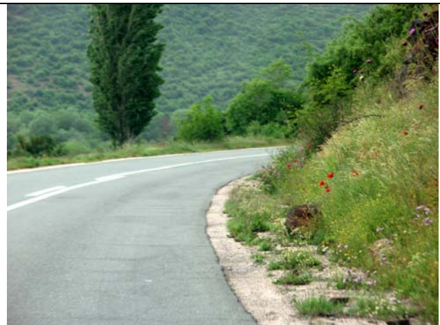
Figure 2.6. Lack of lateral clearance
