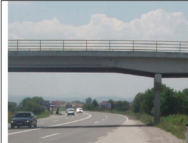
Figure 2.15. Missing guardrail for an overpass bridge pile
