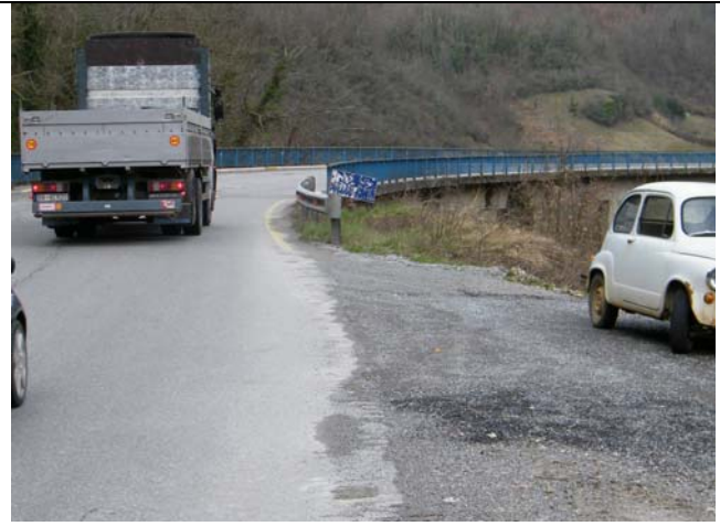
Figure 2.16. Missing guardrail at the bridge section
