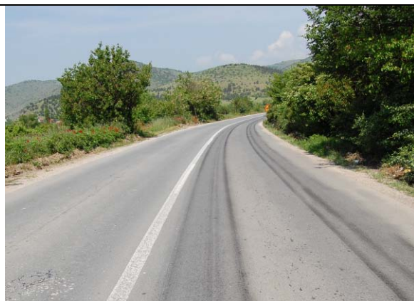
Figure 2.3. Ruttings and bleading of asphalt
